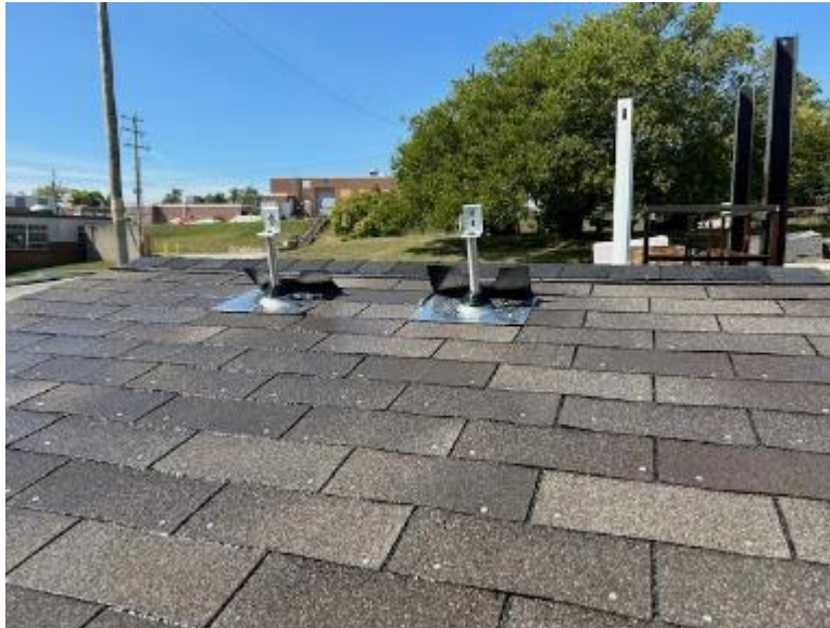
Photo No. 5 70 MPH Top Side
