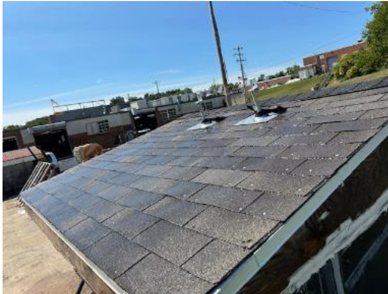
Photo No. 7 90 MPH Top side
