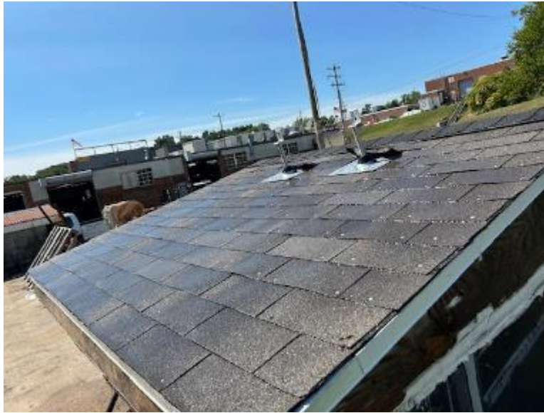
Photo No. 9 110 MPH Top Side
