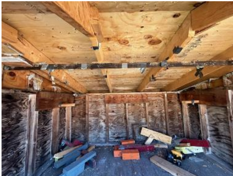
Photo No. 12 Post Test Underside
